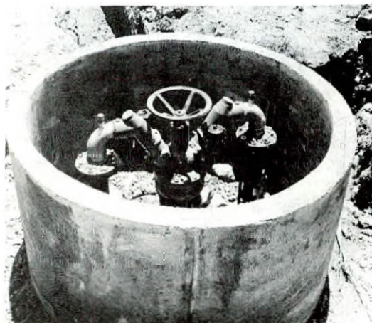
Typical dual outlet farma hydrant of the Paphos Irrigation project.
