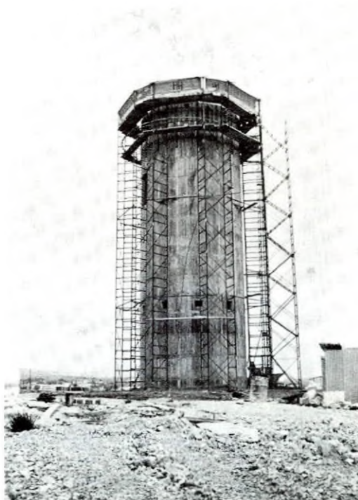
Construction of elevated reservoir in eastern area of Paphos Irrigation Project in progress. Water will be pumped into these reservoirs from the 11.5 km main cannal and from there it will feed the irrigation networks of the valley.
