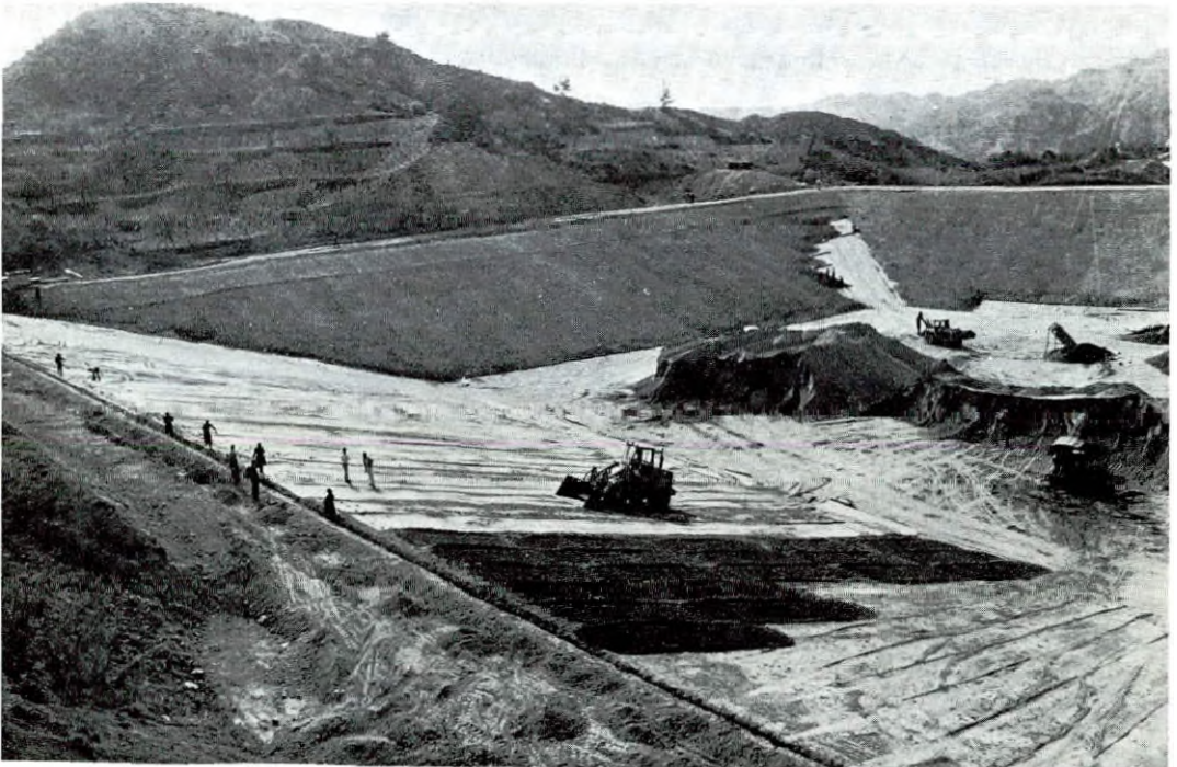
Placing of polythene membrane at Pelendria pond belonging to Pitsillia Integrated Rural Development Project. The 123,000 cubic metres of water to be stored in this pond during winter months will irrigated, together with a borehole scheme, some 480 donums of deciduous trees and vegetables.
