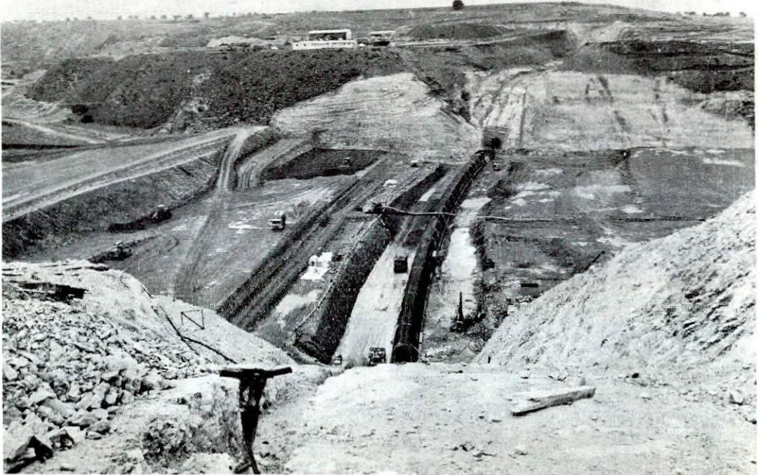
Asprokremmos dam - General view of the dam construction works. The cap gallery over the concrete cut-off wall can be seen along the dam-axis.
