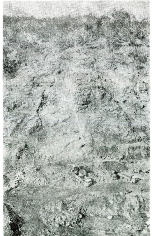
Construction of Xyliatos dam within the Pitsilia Intergrated Rural Development Project started at the end of March 1980. This rockfill type dam will cost approx £1 million and the capacity of the reservoir will be 1.22 MCM. The photograph shows progress in the excavation of the right abutment. WDD Photo 77EN-18 (14.1.81).
