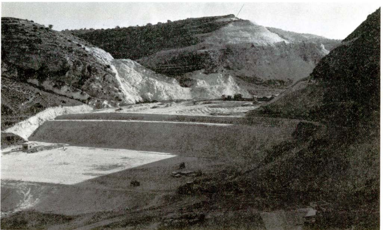
Evretou Dam: Downstream view of embankment with some view of rock quarry in background.
