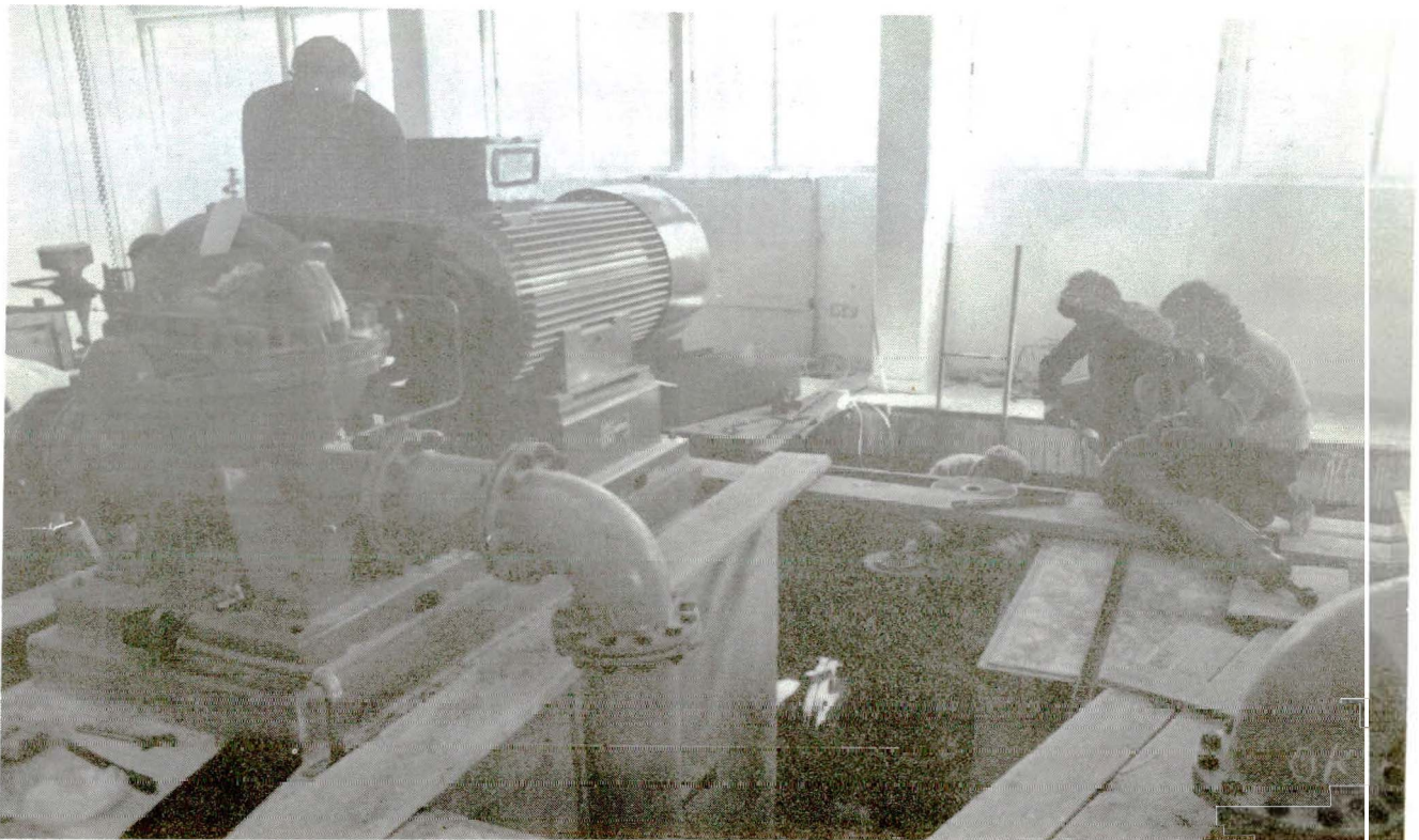
Tokhni Pumping Station. WDD Photo B95EN-6 (6.3.85).
