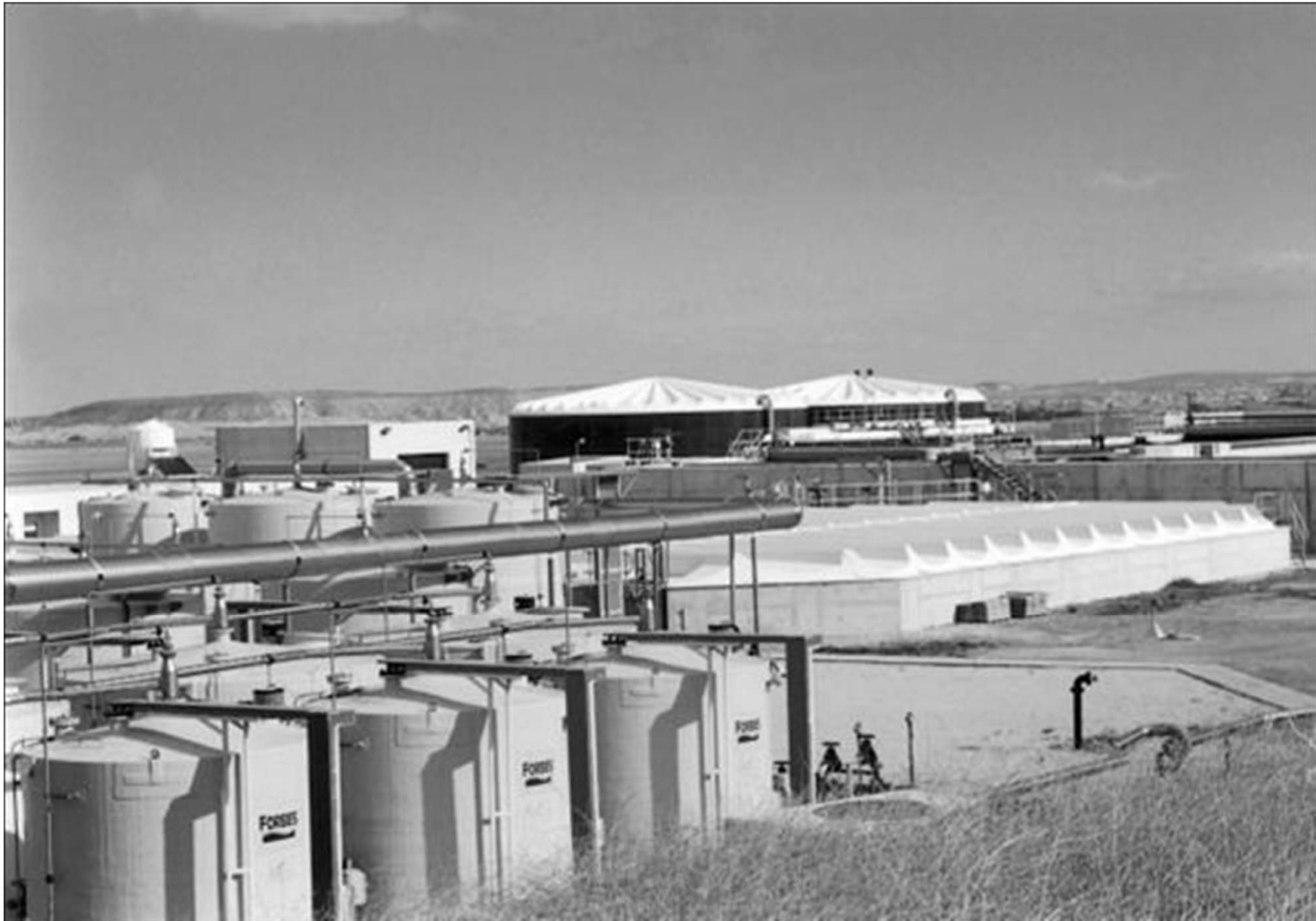
VATHIA GONIA CENTRAL WASTEWATER (SEPTIC SEWAGE/INDUSTRIAL WASTE) TREATMENT PLANT -WDD
