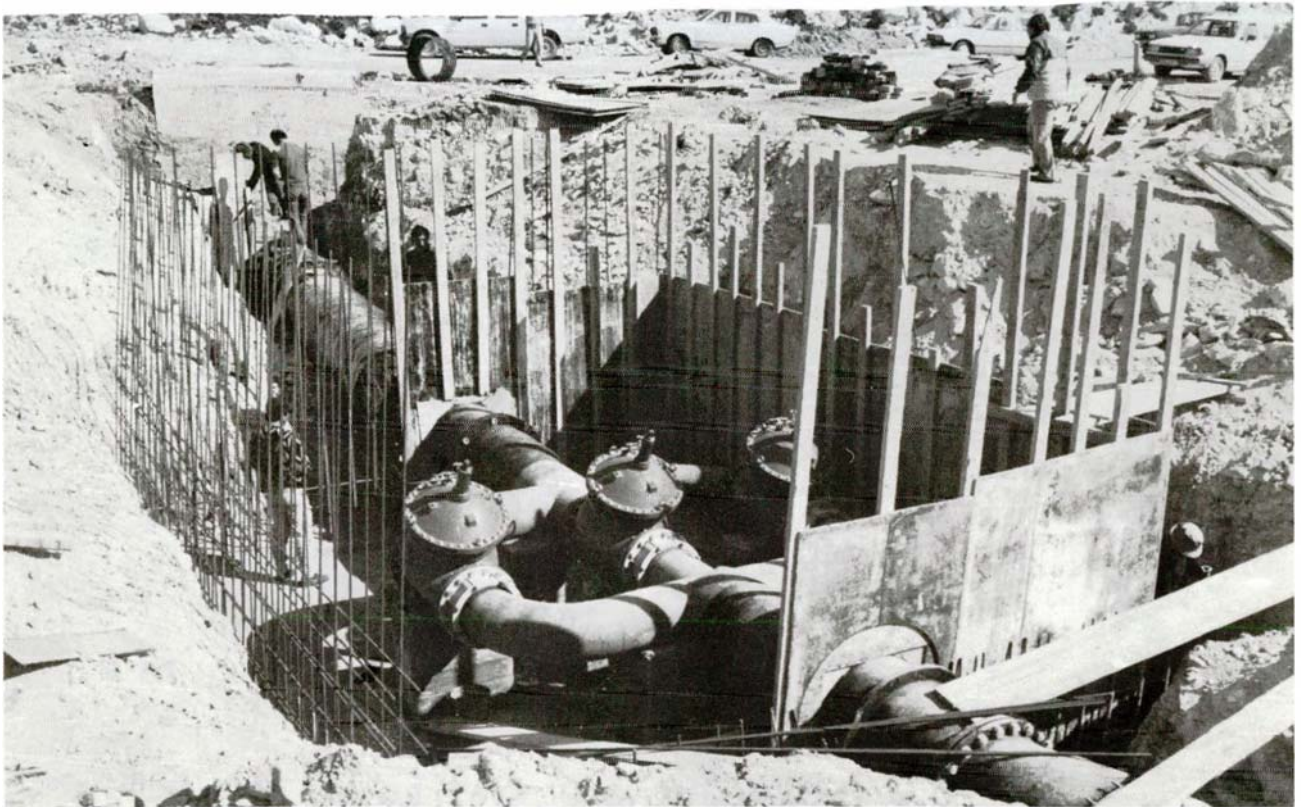
Southern Conveyor Project. Phase II. Akrotiri Irrigation Network. Valve chamber of junction J2 of Akrotiri main pipeline to the Southern Conveyor. WDD Photo F84EN-4 (9.3.89).
